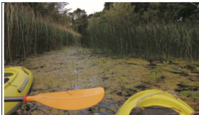
Corbally Canal beyond the (R445) culvert. A densely blocked, silted and almost dead waterway. Weed volumes hold water back, starving supply to the Naas Line. The Greenway here, though a pleasant tranquil walk, will look down upon this decaying monument to poor decision making in Kildare.
